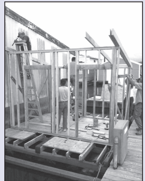
Community volunteers have been donating their time to build floating restrooms for marina tenants.
