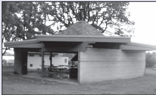
Just in time for summer gatherings, the Scappoose Bay Marine Park’s gazebo has a new roof.
